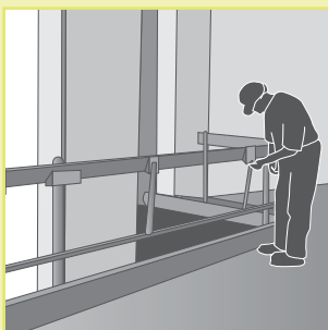
Figure 14: This temporary guardrail is being used instead of mesh to permit work on curtain wall securing bolts.
