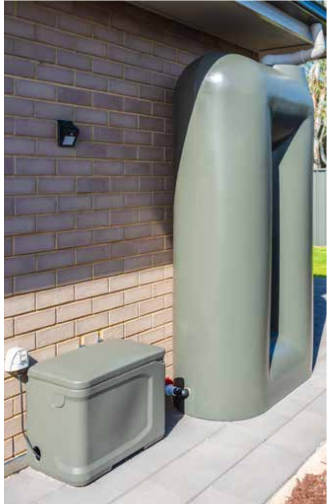
Photo 32: Rainwater harvesting systems should be designed into developments to maximise their efficiency and appearance.
