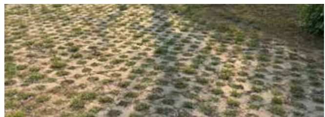
Photo 38: Permeable paving for driveways can effectively manage stormwater, reduce runoff, filter pollutants, mitigate urban heat island and enhance aesthetics.
