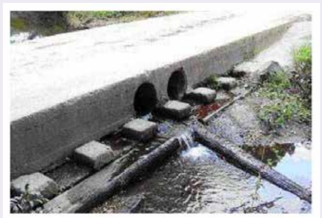
Before & after photos of the same road crossing rehabilitated to allow safe fish passage
