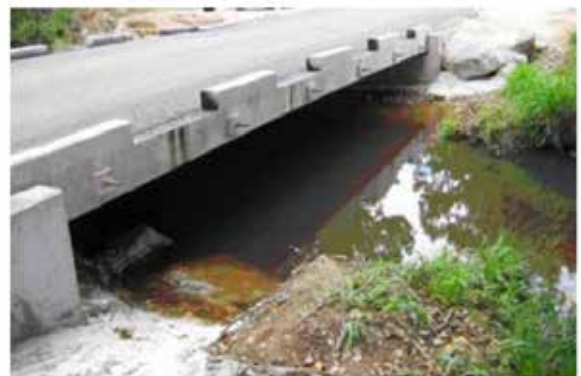
Fauna underpass on the Calder Freeway. Source: VicRoads Fauna sensitive road design guidelines.
